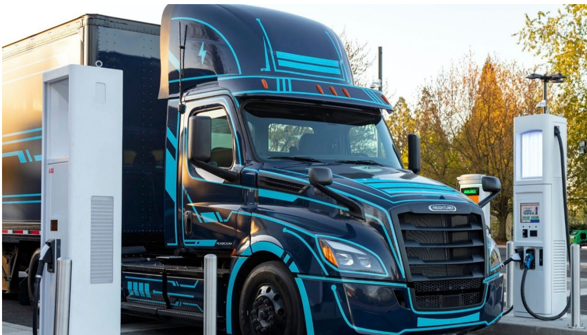
Electric Island: E-Truck charging stations. Photo Courtesy of greencarreports.com 2022.
